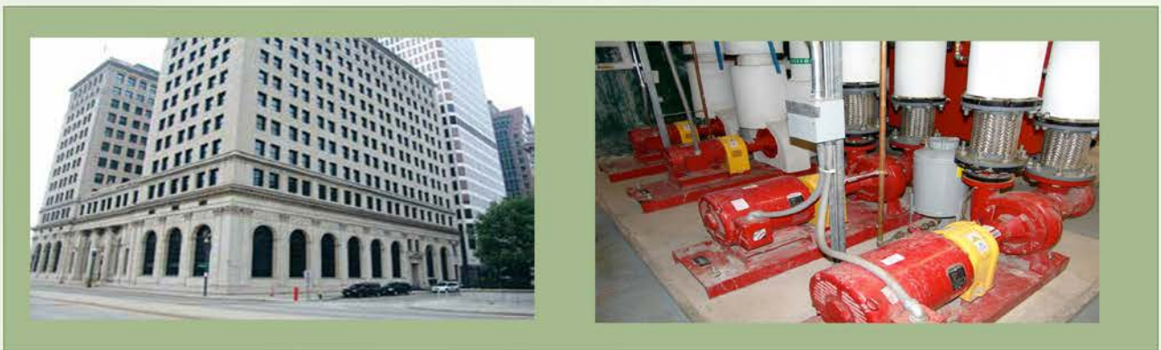
Rhode Island School of Design —EnviroFlo Frame-Mounted End Suction and Vertical In-Line Pumps are maintaining critical climate control requirements in a 128-year-old library while minimizing energy consumption.
