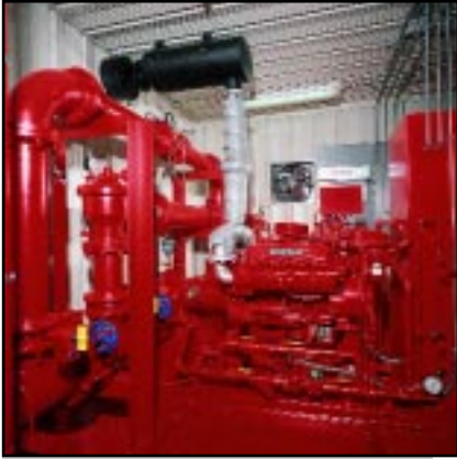
INTERIOR OF A TOTALLY ENCLOSED PRE-PAC.
